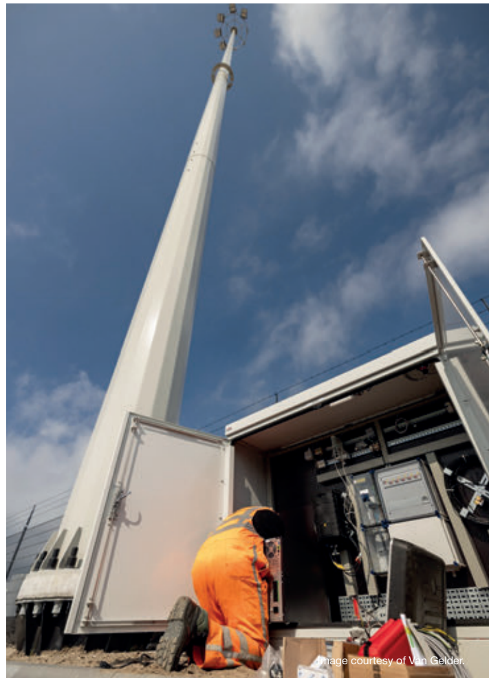
Van Gelder provides comprehensive support in the harbour.
